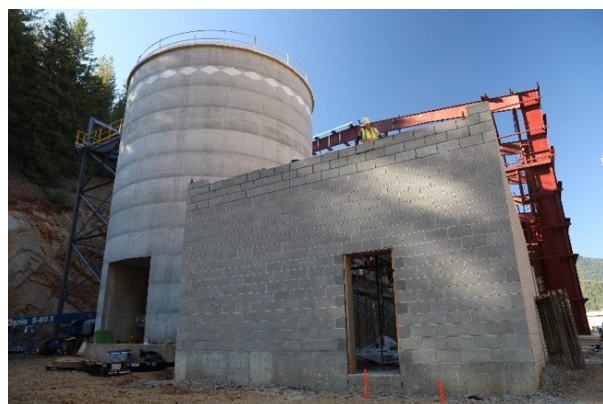
Figure 4: Motor Control Centre Building
