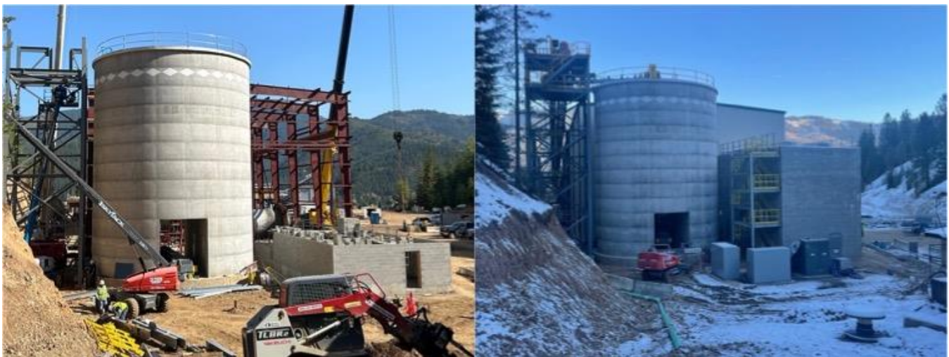
Figure 1: Progress since September 2024 at the rear of the processing facility, ore silo, and motor control center
