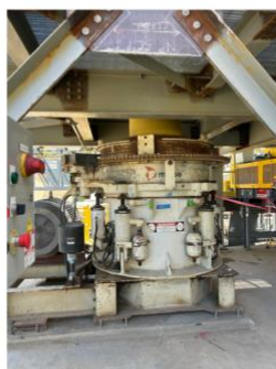
Refurnished Metso Cone Crusher (one of two)
