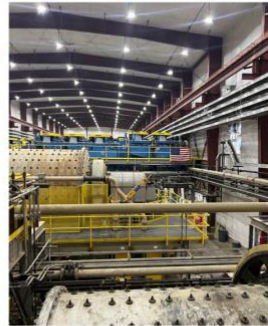
Main and Re-grind Mills in location within the facility
