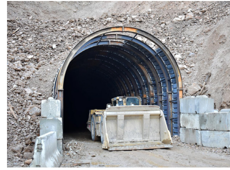
Newly completed and enlarged Russell Portal to support expansion up to 2,500 tpd
